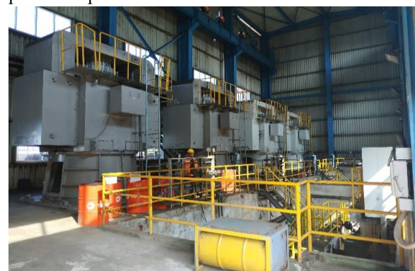
Figure 3. Fire-Resistant Construction at Pacitan Steam Power Plant, East Java, Indonesia. Source: Pacitan Steam Power Plant, 2025
